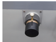
Cooling coil collector pipe
